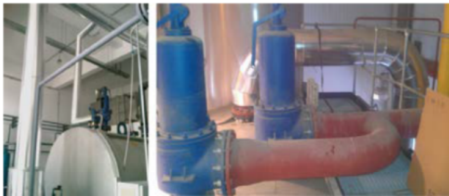
Fig. 16 Impermissible merging of safety valve and expansion steam pipe
