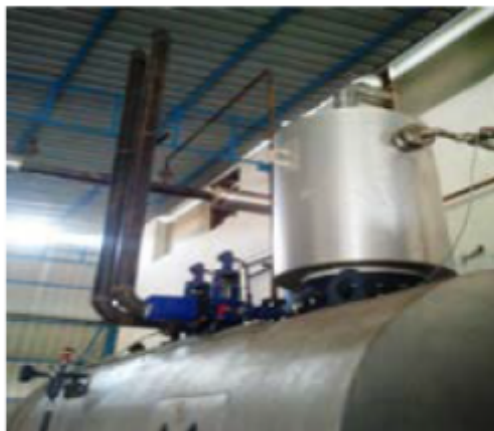
Fig. 20 Holders of safety valve blow-off pipes missing
