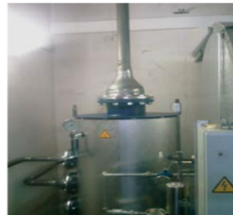
Fig. 17 If the internal diameter of expansion steam pipes is reduced, this can lead to an increase in pressure and rupturing of the vessel
