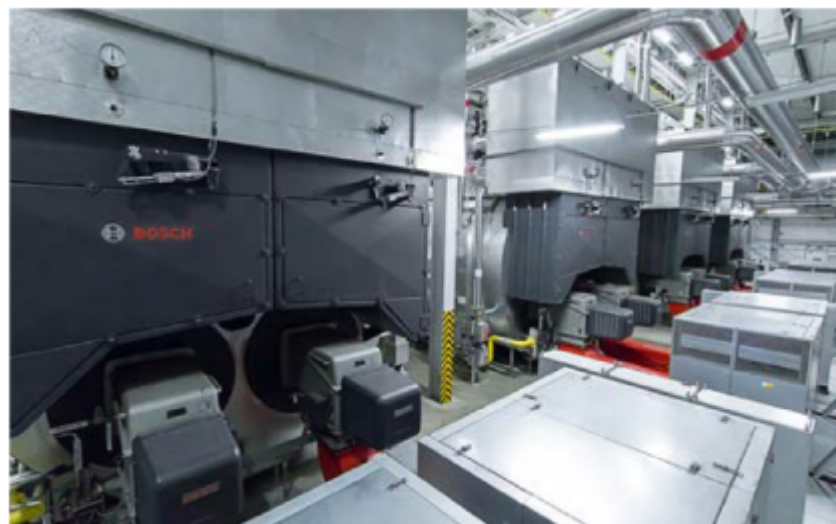
Fig. 73 Double flame-tube boiler with mounted superheater on top
