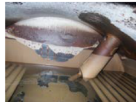
Fig. 23 Water-side deposits on the tube panel and tube plate of the boiler
