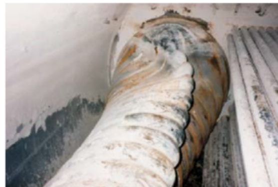
Fig. 90 Layer formation in boiler with damage to flame tube
